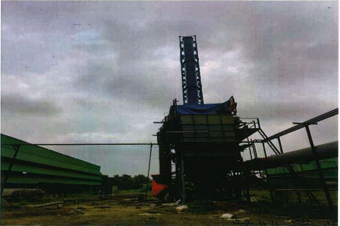
Zinc Spray painting Cyclone with Bag filter and Chimney.
